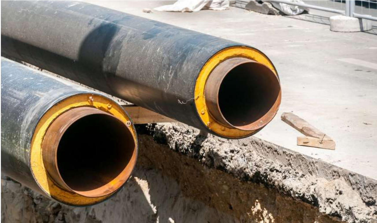
DISTRICT HEATING NETWORK
